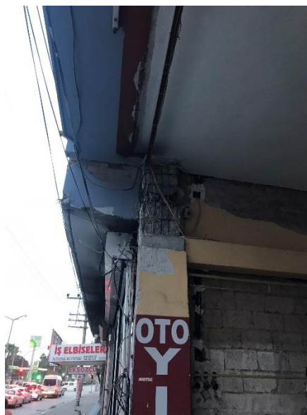
Figure 8. Short column damage
