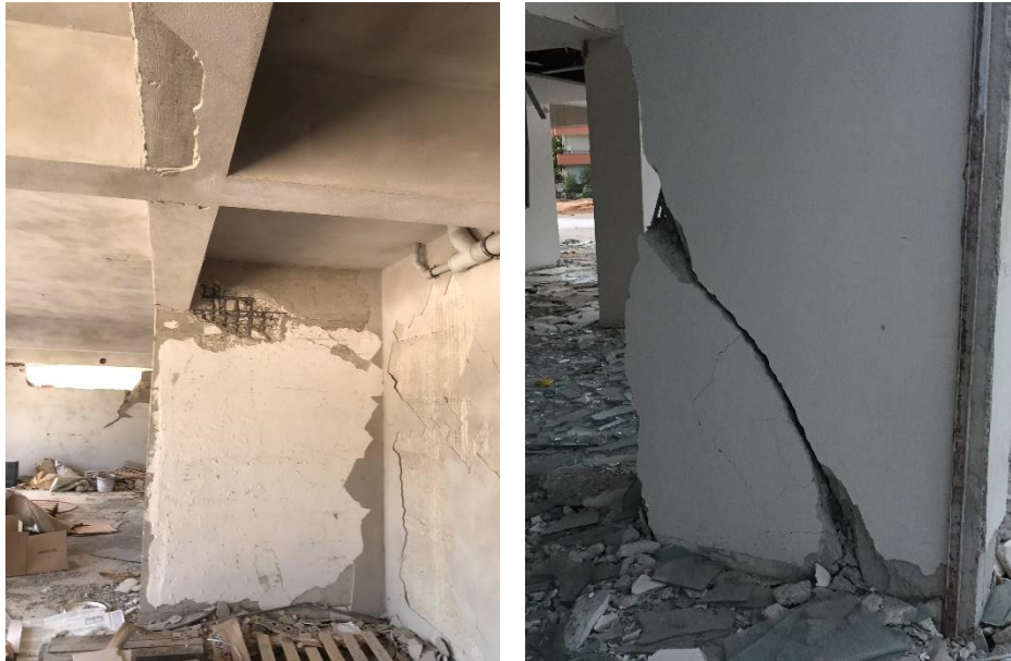
Figure 7. Reinforced concrete shear wall damage
