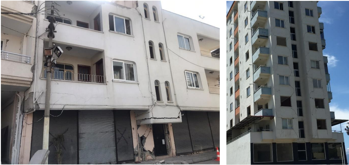
Figure 5. Long cantilever and overhang damage
