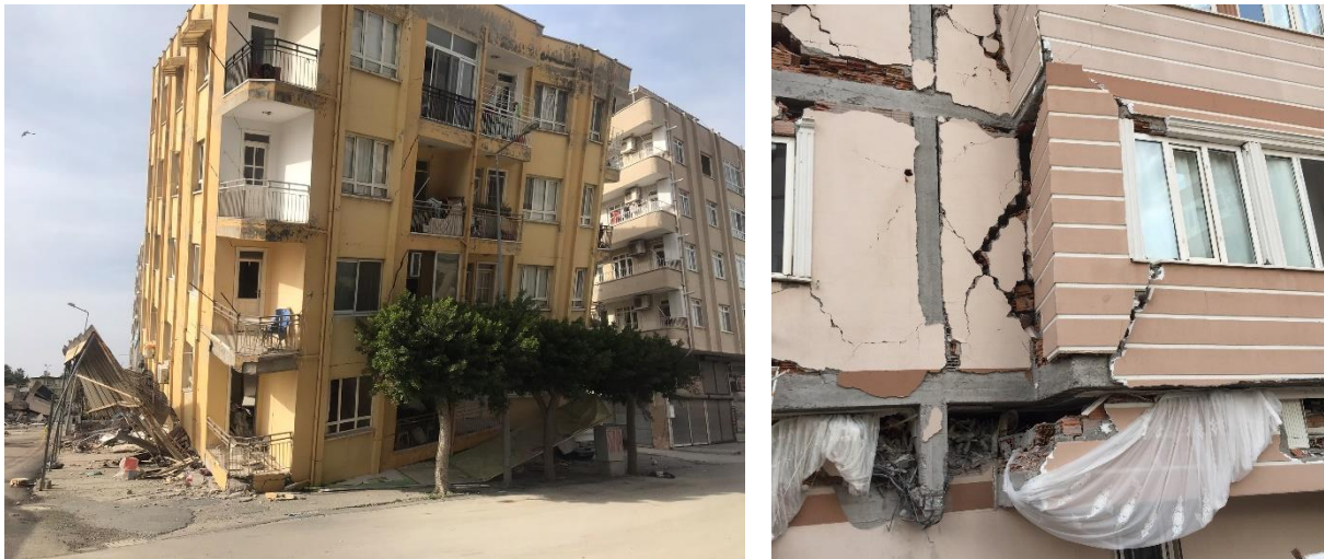
Figure 9. Soft/weak story damage
