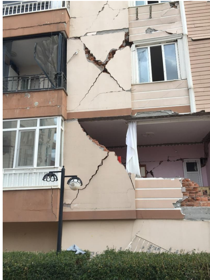
Figure 4. Infill wall damage
